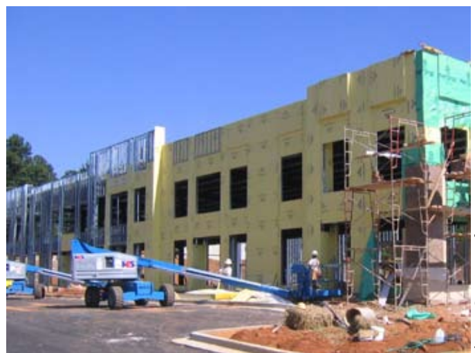
Facade of Commerce Park at Northbrook, showing the installation of Georgia-Pacific Gypsum's DensGlass sheathing.
