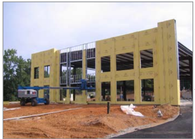
Georgia-Pacific Gypsum's DensGlass sheathing as seen in the construction phase of the new Commerce Park at Northbrook, an office condominium project in Suwanee, Georgia. Project architect and developer - Kenneth Klebanoff, AIA, LEED AP of Trylon Architects.
